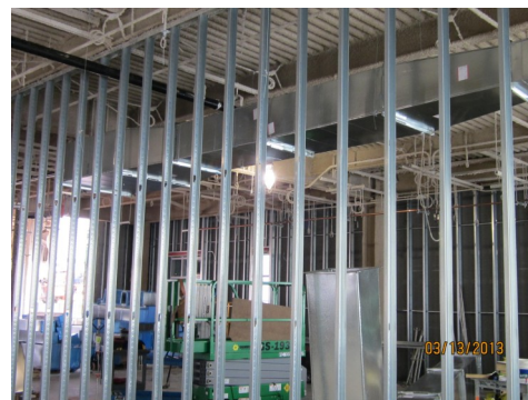
Above; Metal studs and duct work are being installed on the 2nd floor of area D. This room will also be the location of the initial lab mock-up.
