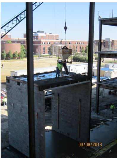
Bellow; Concrete workers place and finish concrete at the main vestibule in Area B. The top of the vestibule required a few yards of concrete to be placed over 25 feet above finished floor.
