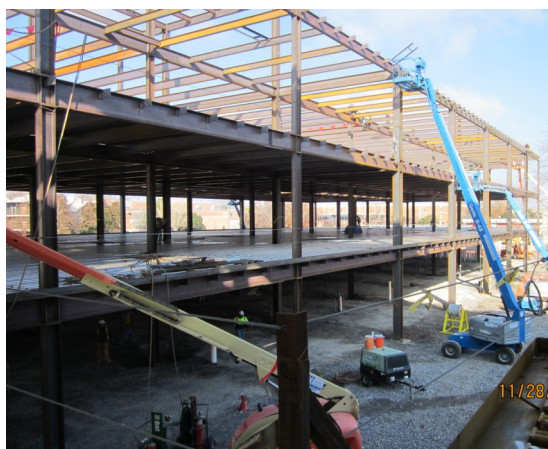
Above: Steel workers erect areas C and B steel. This picture is from the West end of area D looking at the East side of area C
