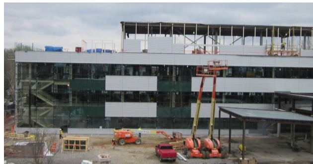
Above; On the North side of Area D the glass and metal panel curtain wall nears completion. In the penthouse of Area D workers install the metal panel system that will enclose the area.
