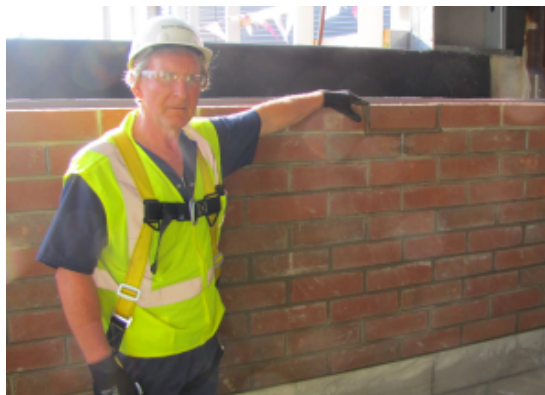
MTSU and TBR Representative Earl Bogle lays the last brick on the interior wall in the A/B connection.
